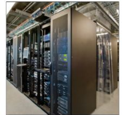
Server towers with racks
